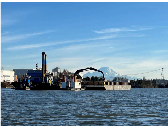
Dredging operations at SMA 9 with Mount Rainier in the background (January 16, 2026, Geosyntec).
