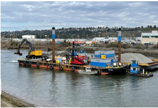
The contractor placing clean material for cap at SMA 12B, after dredging is complete. (King County, February 2026).
