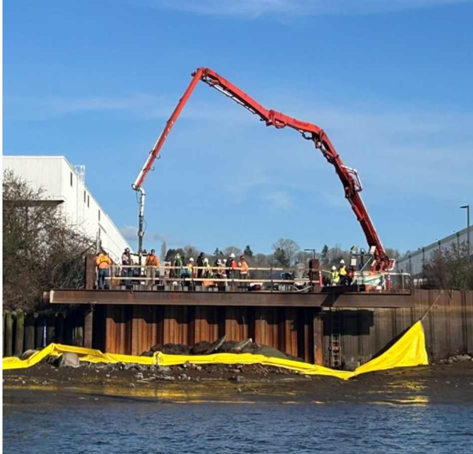
Placing concrete to finish the SMA 9 bulkhead wall system (sheet pile wall) (Geosyntec Consultants, week of March 3, 2025).
