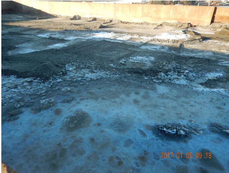
Photo 1-A: Cold weather froze water and ENR material in the barge. Excavator was used to break up the frozen ENR material prior to placement.
