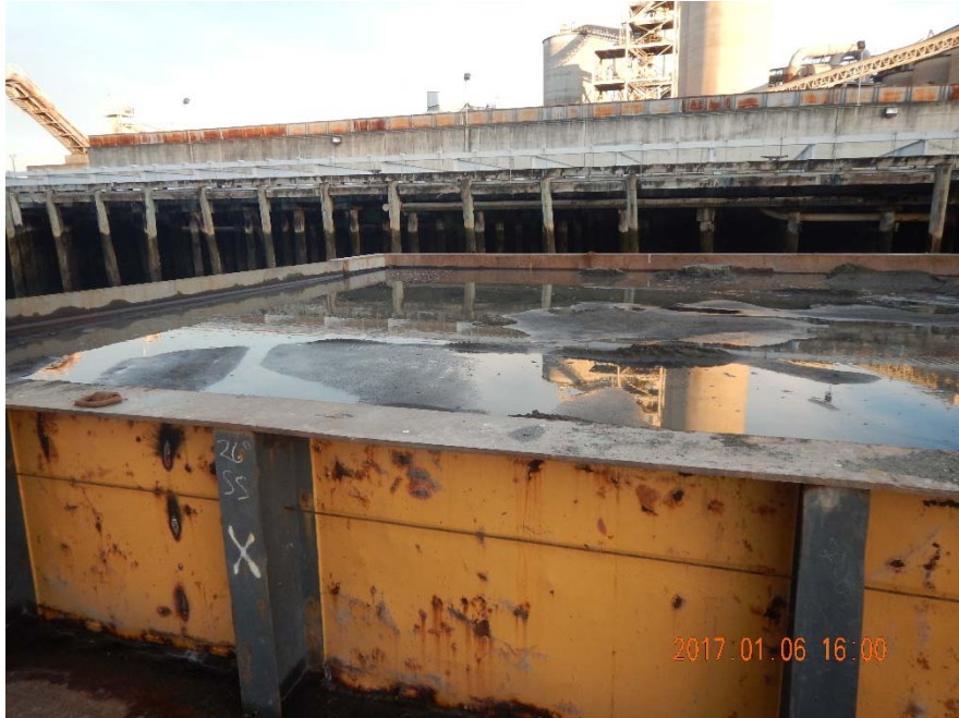
Photo 2-A: Soaking of the Sand+AC ENR material. Material was soaked over the weekend prior to mobilization to the Subtidal Plot.
